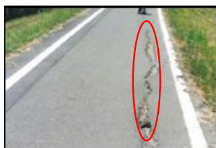
堤防天端の亀裂
