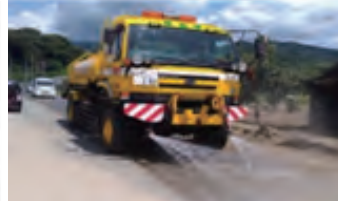
Removal of sediment deposited on road surfaces (2017 Heavy rain in North Kyushu)
