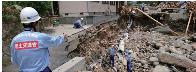
Implementation of investigation of the disaster situation of collapsed roads (2017 Heavy rain in North Kyushu)
