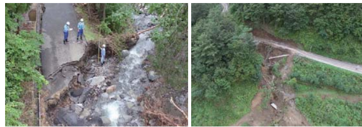
Surveys of damaged roads (Typhoon No. 10 Torrential Rain in Tohoku in September 2016)
