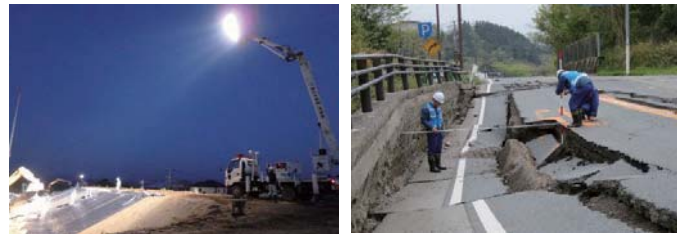
Emergency construction assisted by lighting car (April, 2016 Kumamoto Earthquake) Investigation of road damage area
