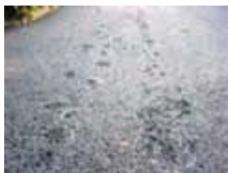
舗装表面の骨材飛散
